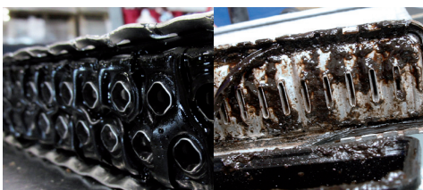
Figure 1: Rubber seals degraded by oil
