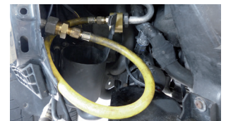
Figure 2: Filter-driers/accumulators should be bypassed and replaced before flushing.
